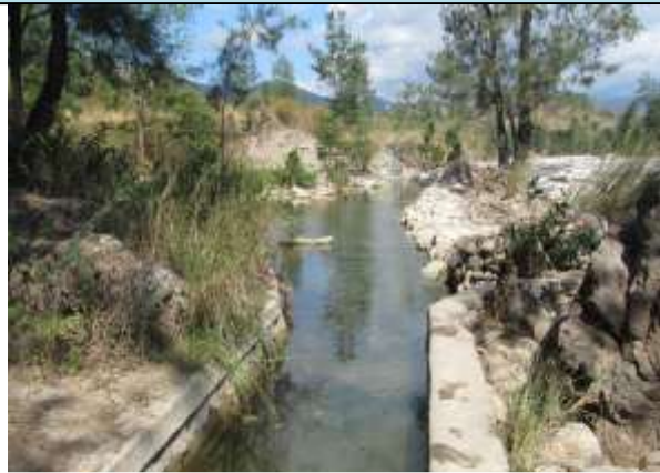
Irrigation systems in Kuateles that were built during the Indonesian occupation still greatly benefit locals, but the Timor-Leste Government needs to fix them further (image: LH).
