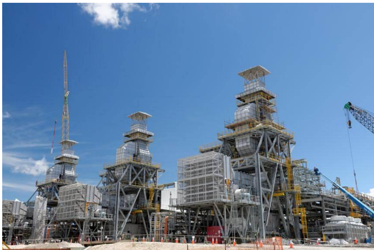
Hides Gas Conditioning Plant, PNG LNG, September 2013.
