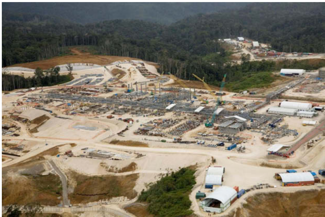
Hides gas conditioning plant, December 2012
