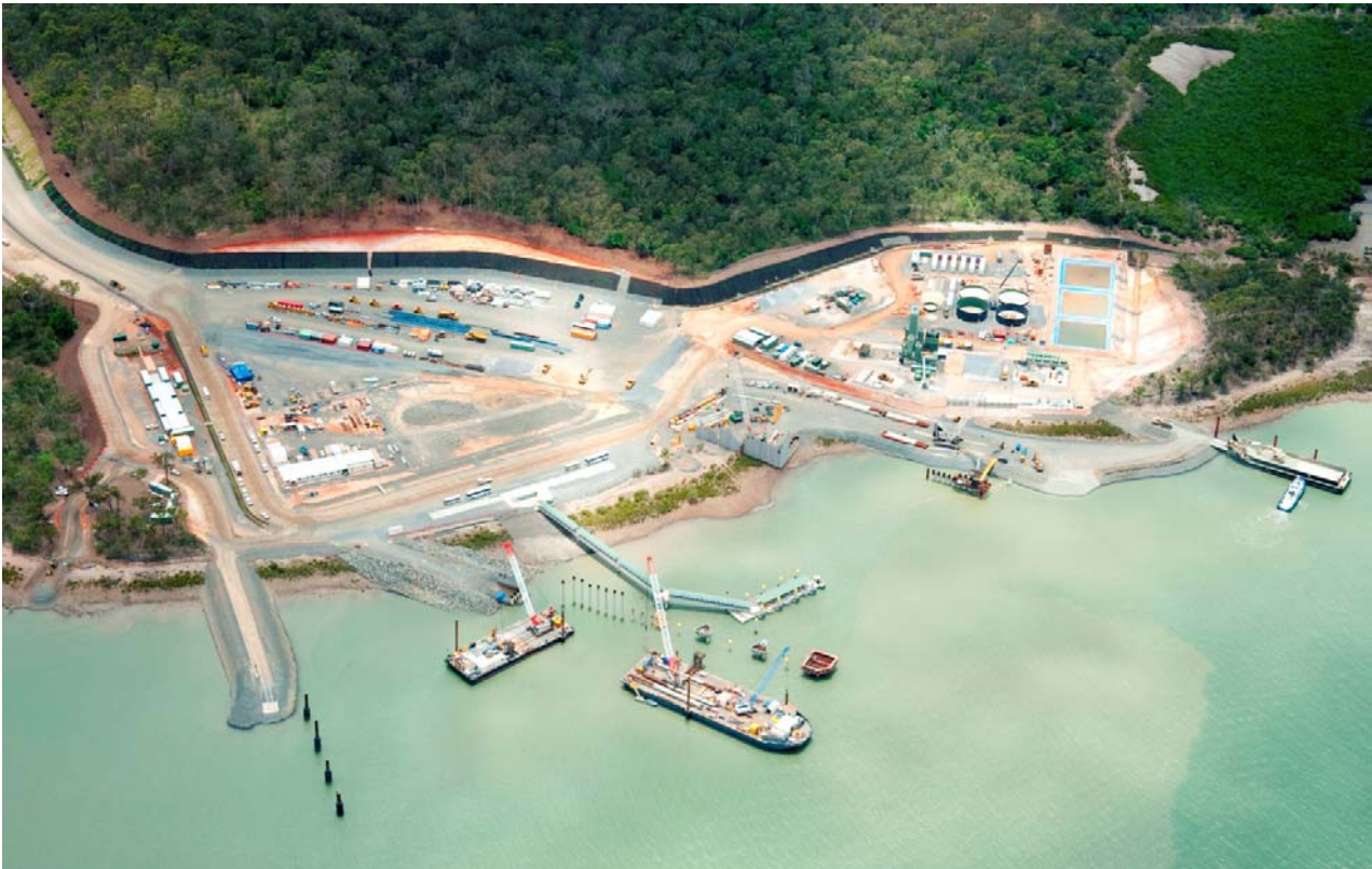
Aerial view of the GLNG material offloading facility site on Curtis Island, 3 January 2012.
