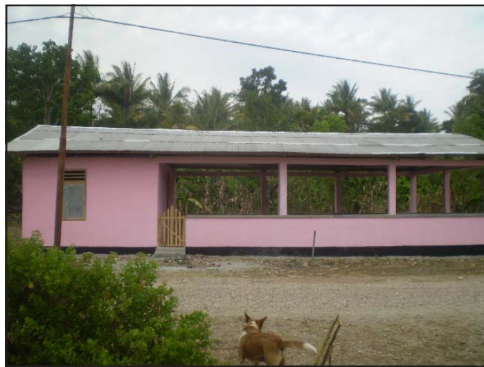
CDF project in Abani village. This community meeting building was finished in August but has not been in use since because construction workers have not been paid and are withholding the keys.
