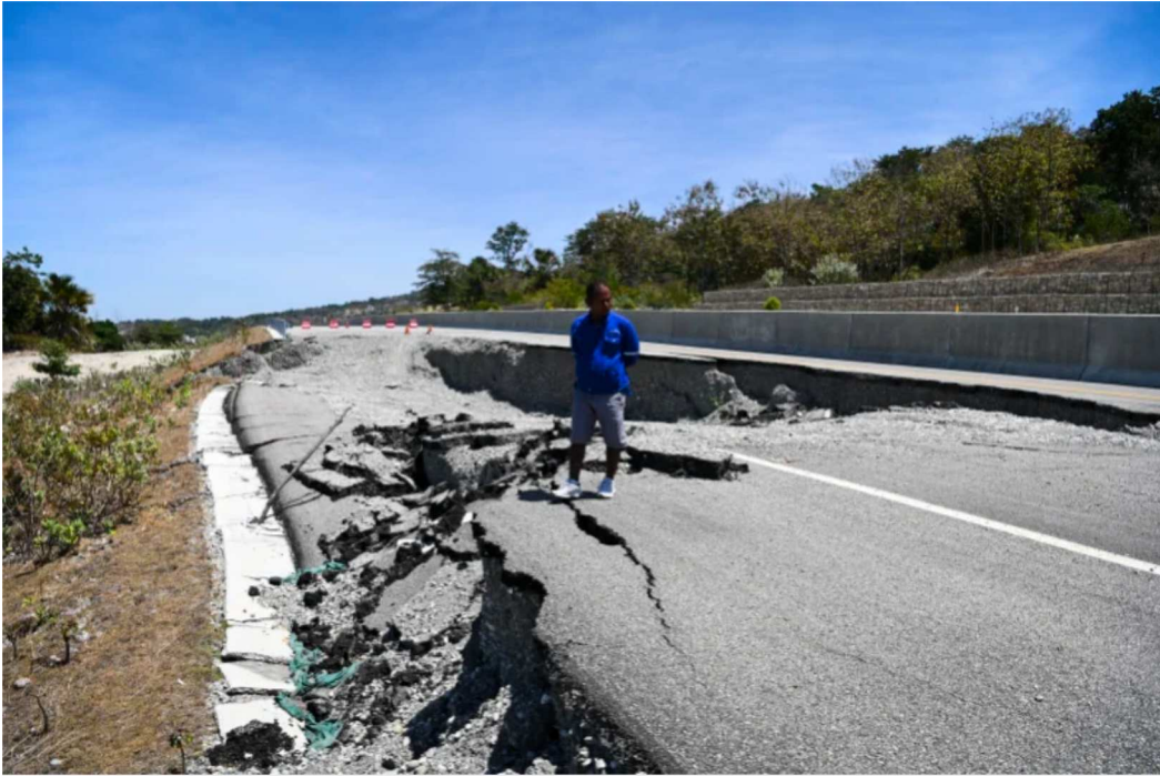
A severely damaged section of the Suai-Fatucai expressway built by Covec-CRFG (joint venture between China Overseas Engineering Group Co. and China Railway First Group Co.) AAP IMAGE/LUKAS COCH
