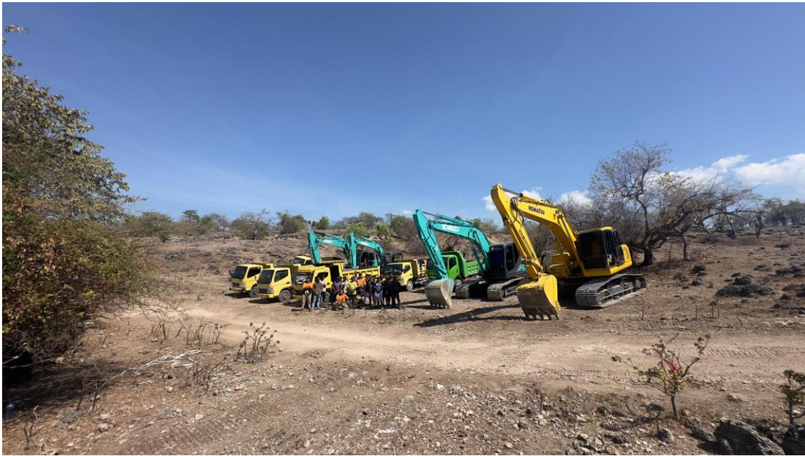
Figure 8: Mobilisation day of contractors to the Werumata Limestone Project to commence drill track and pad preparation.
