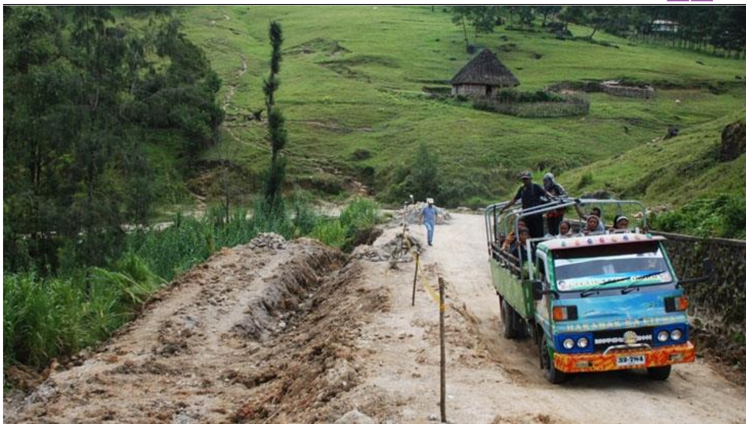
FIGURE 4.6 EXAMPLE OF POOR ROAD SECTIONS IN TIMOR-LESTE
