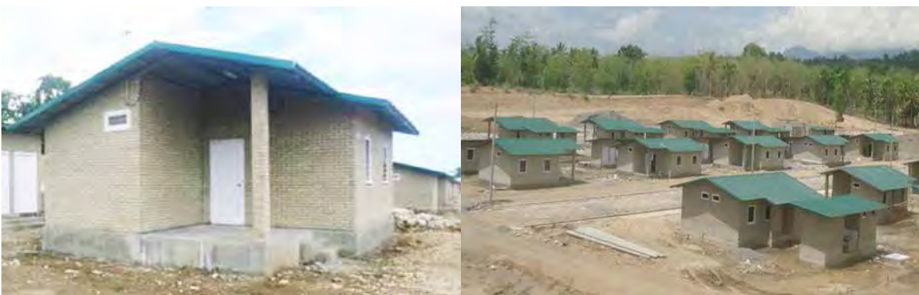
Construction progress of the infrastructure facilities for the support of Suai airport
