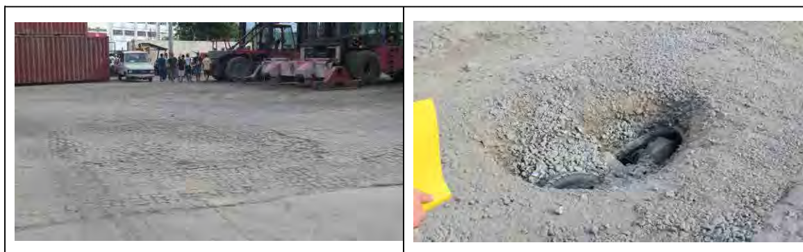
Figure 1.2-5 Deterioration Area of Pavement and Cave-in Point
