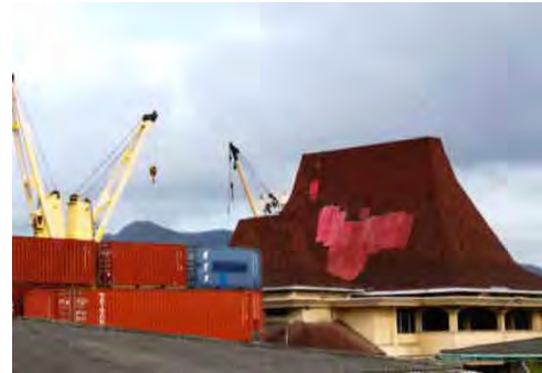
Figure 8.2-4 Badly Damaged Passenger Terminal Building (under repair)
