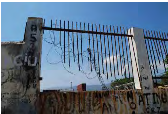
Figure 1.6-11 West Fence (Eroded Area)
